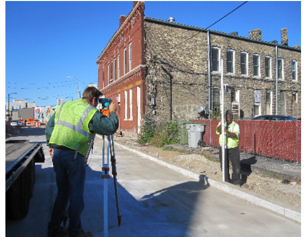
Above: Resident Engineer Steve Graetz works with James Boyd just south of Mitchell preparing for the installation of the east sidewalk.
