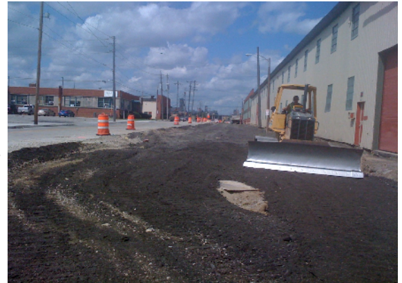
Crews from Zignego Construction are working to level, grade, compact and place crushed stone prior to new concrete being poured.
