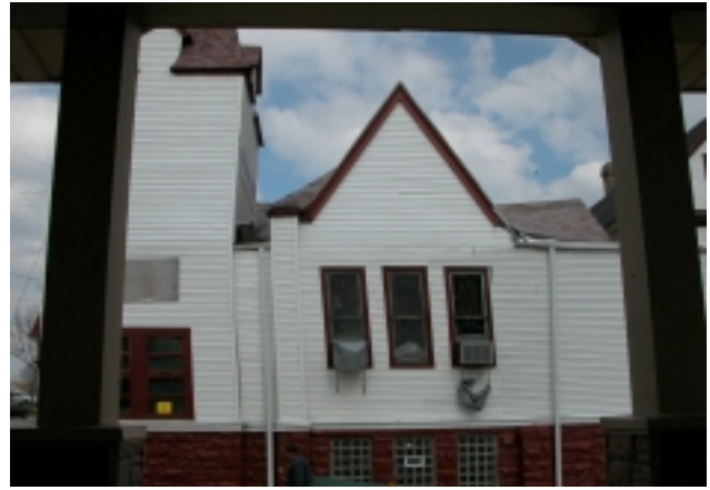
The bend in the steeple is most noticeable when the vertical columns left and right show the amount of tilt in the building.
