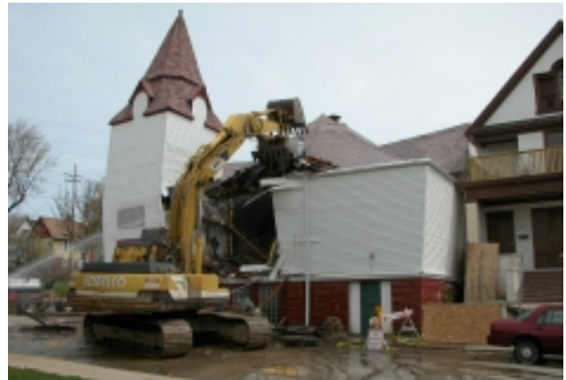
Here the wrecking machine is carefully peeling off the roof in hopes the steeple will fall into the center and not shift the building southward.
