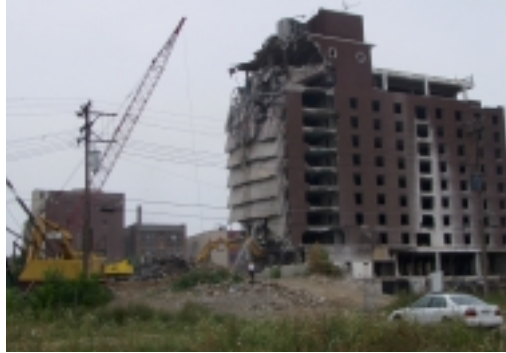
Demolition is started on the former Holiday Inn located at 2601 W. Wisconsin Ave.
